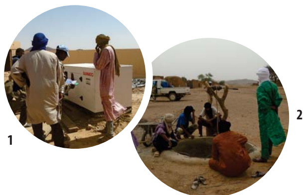
Views of works in progress in Tessalit by ADMSM NGO (Association pour le Développement Multi-Sectoriel au Mali):
