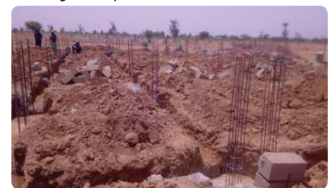
Construction site of the sheep breeding infrastructures in the prison in June 2016
